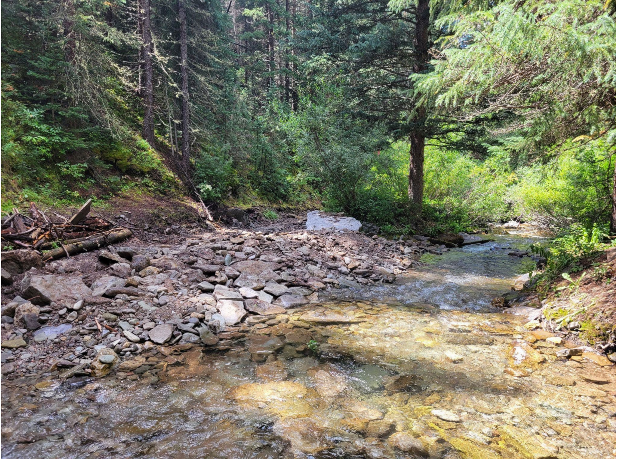
Figure 4. Same stream crossing as Figure 3, after road maintenance was completed in Aug. 2022. The road prism was raised on each side of the crossing to prevent water from running down the road.
