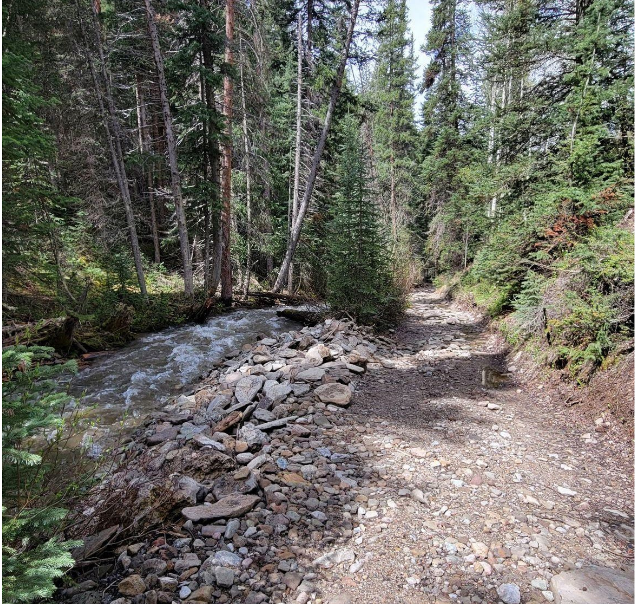
Figure 2. Example of the co-location of Wearyman Creek and FS Road 708.1. Photo taken May 2023, after road maintenance was completed in Aug. 2022. Even with the armoring and raising of the road/stream bank, some water is still flowing into the road prism.
